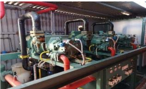
INDUSTRIAL REFRIGERATION SYSTEMS
